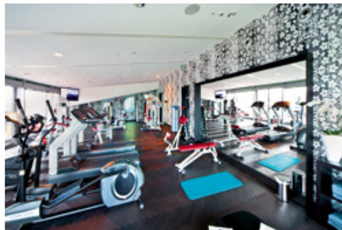
Caption: Be it testing your stamina or simply toning up, jet nozzles from TROX supply fresh air in the fitness area
