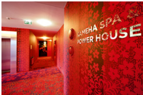
Caption: Fire protection valves from TROX also provide safety in the hallways
